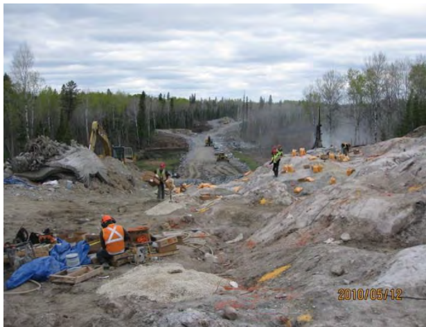
Photo 3: Crews prepare a site for blasting after all required licences, permits and certificates are obtained.
