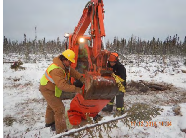
Photo 2: Contaminated soil being placed in a hazardous materials bag along transmission rights-of-way (ROW).
