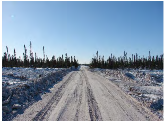
Photo 4: An access trail constructed on frozen ground to minimize ground disturbance and rutting.
