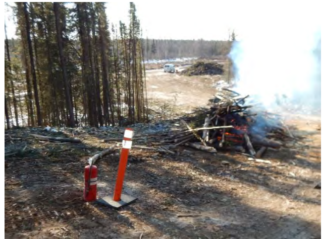
Photo 2: A fire extinguisher is marked and located near a burning pile.
