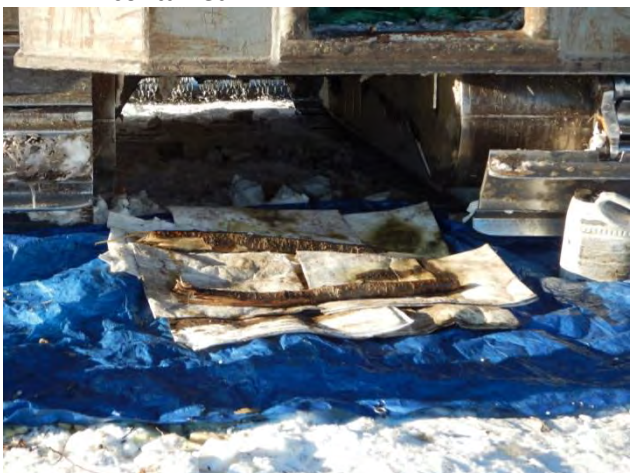
Photo 6: Spill pads to soak up an oil leak.
