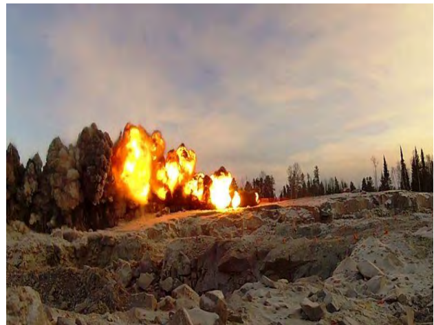
Photo 4: Blasting occurring outside of timing windows for sensitive bird breeding, nesting and brood rearing.
