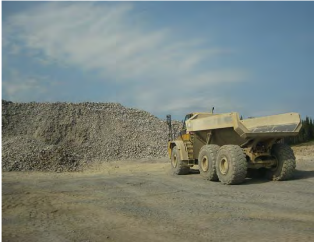
Photo 1: Gravel from a borrow pit being loaded onto a truck for transportation.
