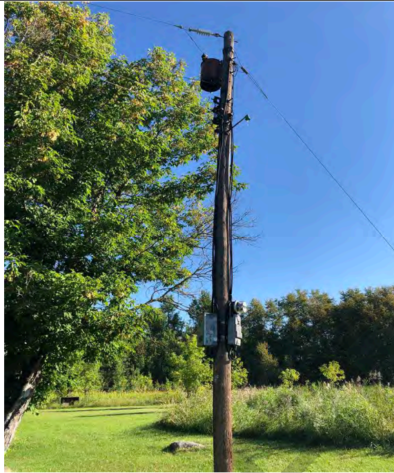
Photo 7: August 30, 2022: Facing northeast showing the power pole with pole-top transformer and auxiliary electrical equipment in the west portion of the site.
