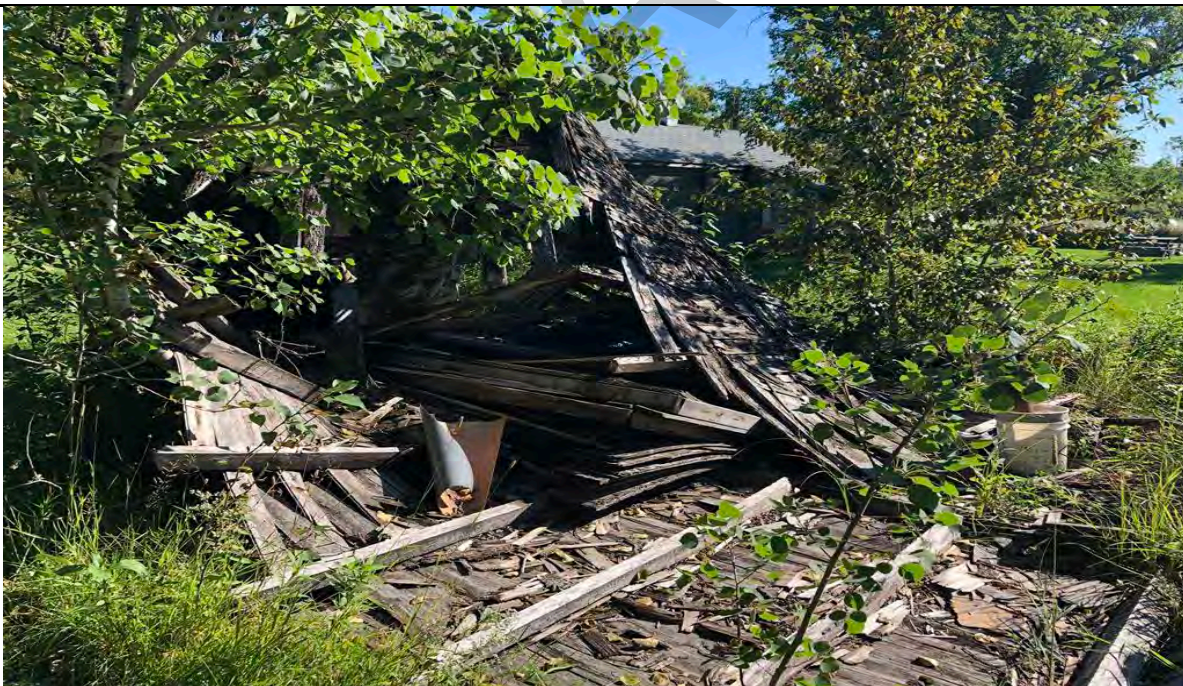
Photo 8: August 30, 2022: Facing north showing a collapsed wooden shed in the west portion of the site. Various debris and metal scraps are visible.
